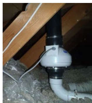
Figure 4. Blower installation inside attic, outside occupiable building envelope. Source: Clean Vapor, LLC
