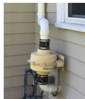
Figure 3. Blower installation outside building. Source: C. Regan, ERM
