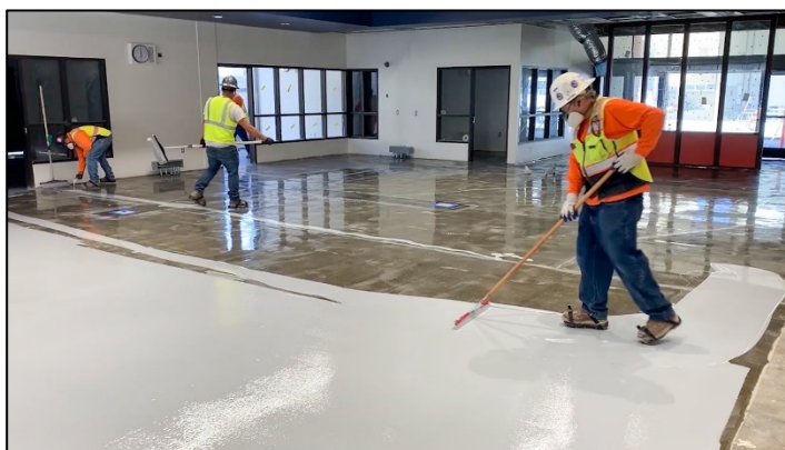
Figure 1. Application of EFC to a concrete substrate. Source: Land Science, a Division of Regenesis, used with permission.
