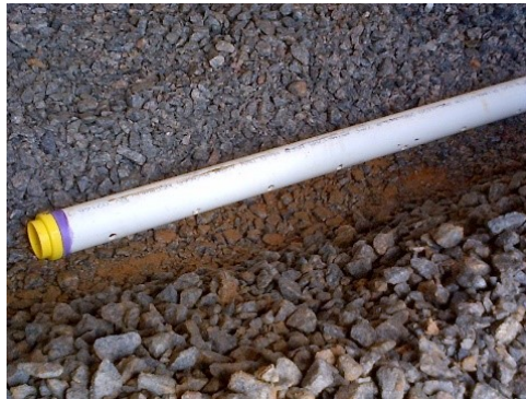
Figure 4. Photograph of mitigation system piping.
