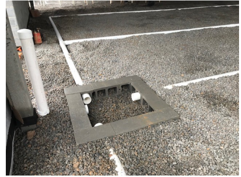
Figure 5. Photograph of a header for mitigation system piping.
