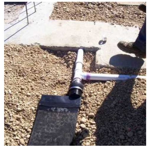
Figure 3. Photograph of a low-profile vent and vent pipes.
