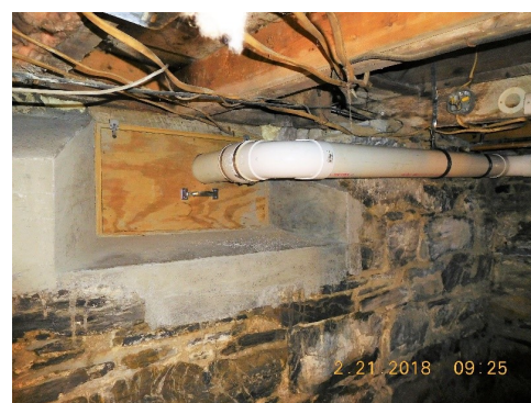
Figure 2. Example piping into a crawlspace area.
